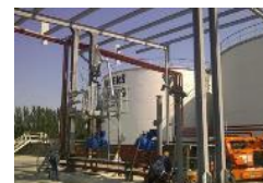
Pumps and compressors
